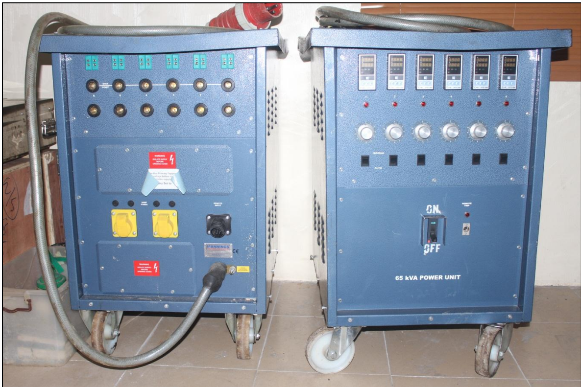
Post Weld Heat Treatment Machines.
